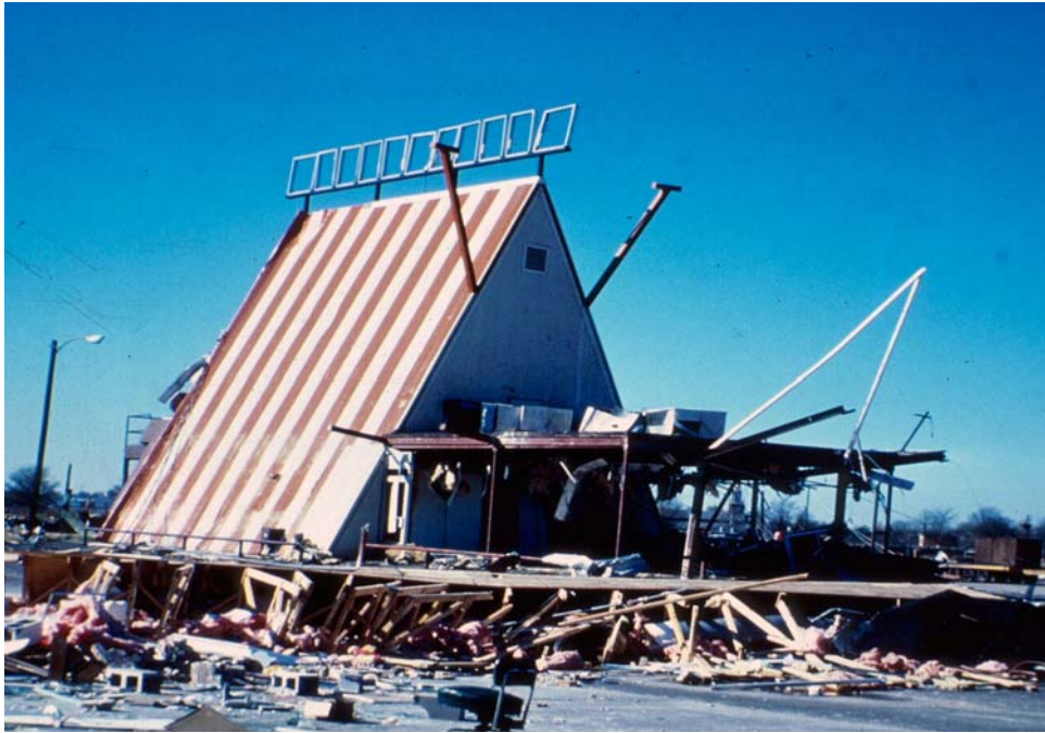
SRB: DOD 5: Canopies and covered walkways destroyed
