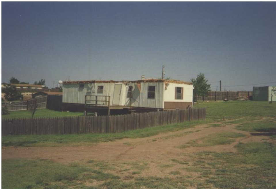
MHSW: DOD 4: Complete uplift of roof; most walls remain standing
