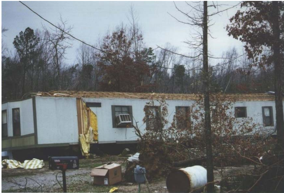
MHDW: DOD 5: Uplift Of roof deck and loss of significant roof covering material (>20%)
