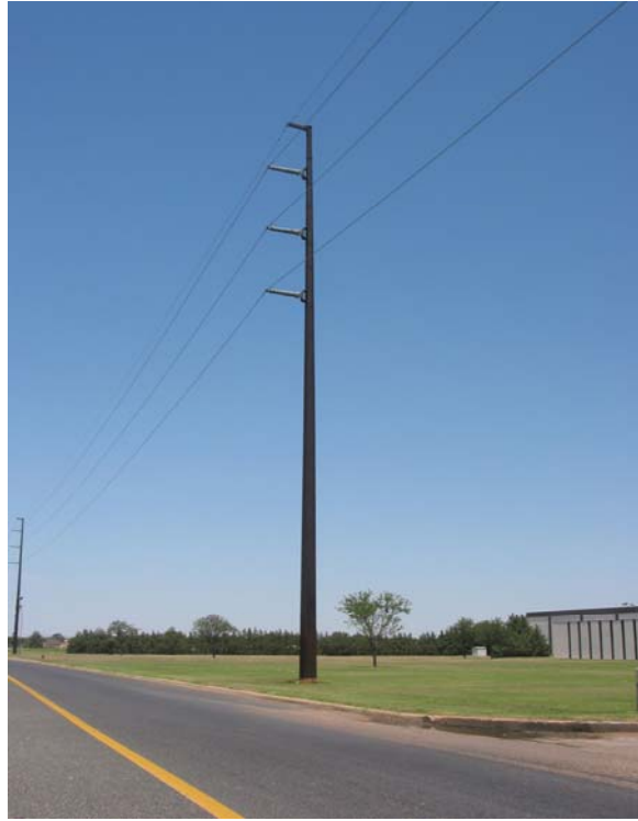
ETL: Single Steel Pole
