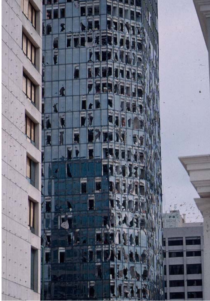
HRB: DOD 5: Broken glass in curtain wall; significant damage to building interior
