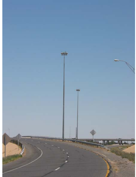
FSP: Luminary Poles
