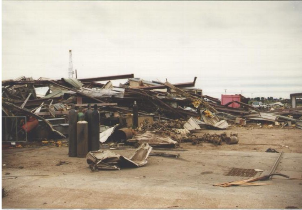
MBS: DOD 8: Total destruction of building
