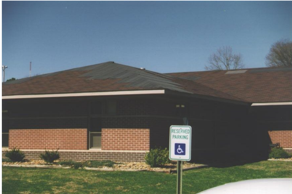
FR12: DOD 2: Loss of roof covering (<20%)
